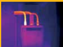
Poor connection and internal damage
