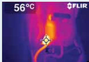
What a thermal imaging camera sees.
