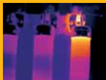
Internal fuse damage
