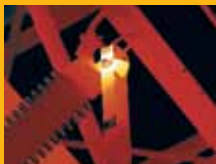
Incorrectly secured connection
